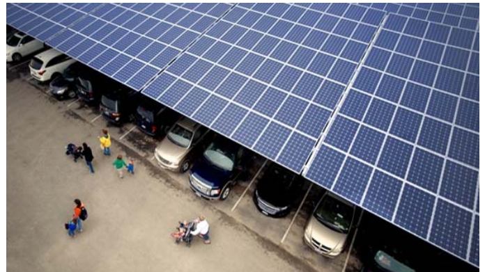
A huge solar power array over the parking lot supplies 20% of the Zoo’s electrical needs.
